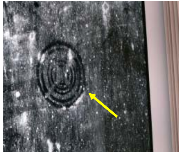
Photo Above shows an installed window with heavy condensation on Glass. Different patterns are visible within the condensation including the outline of a Suction Cup mark which may have been used to handle the glass during fabrication or installation. There are no visible marks present on this glass in the absence of condensation.
